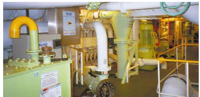
The compact OptiMar system installed on the Regal Princess
