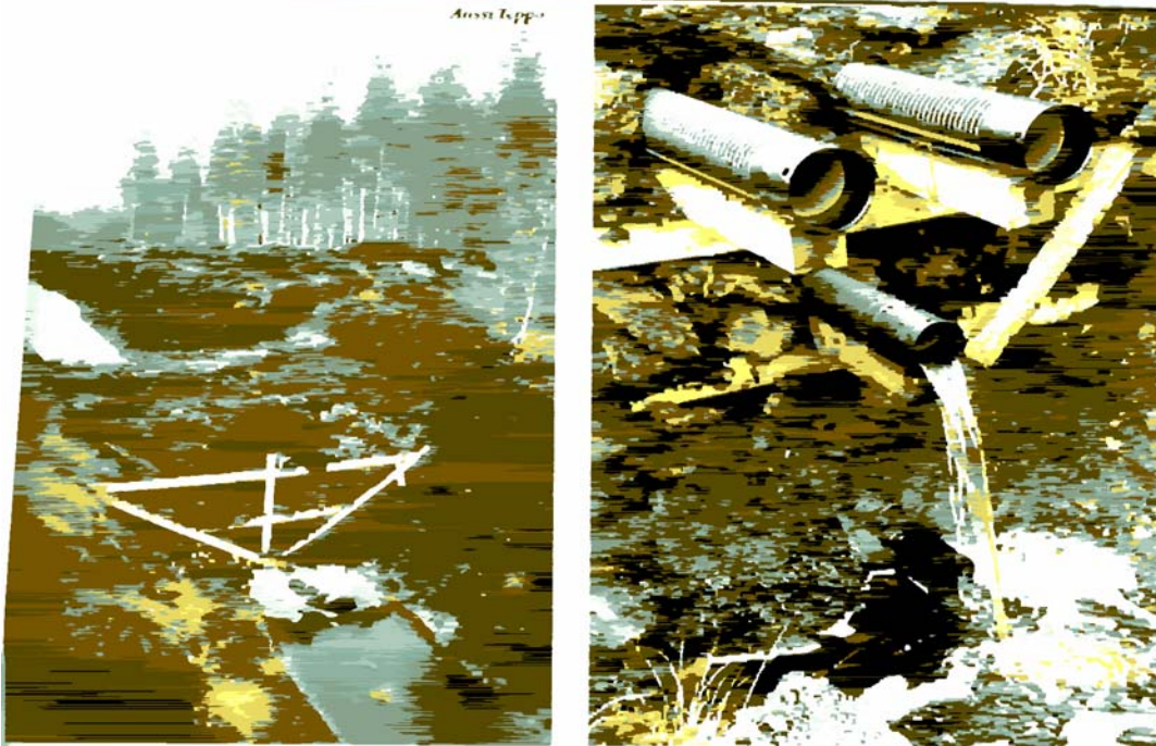
During times of low water flow all drainage waters will run out through the lowest pipe of the dam.
