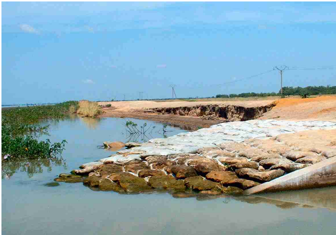
Photograph 1: erosion of upstream shoulder
