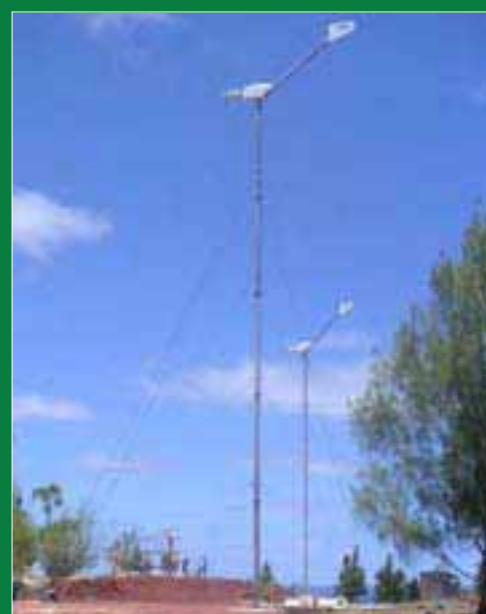
A wind resource turbine for energy production in Mangaia, Cook Islands.
