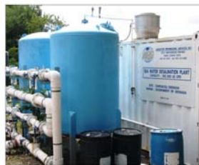
Desalination Plant, Carriacou, Grenada
